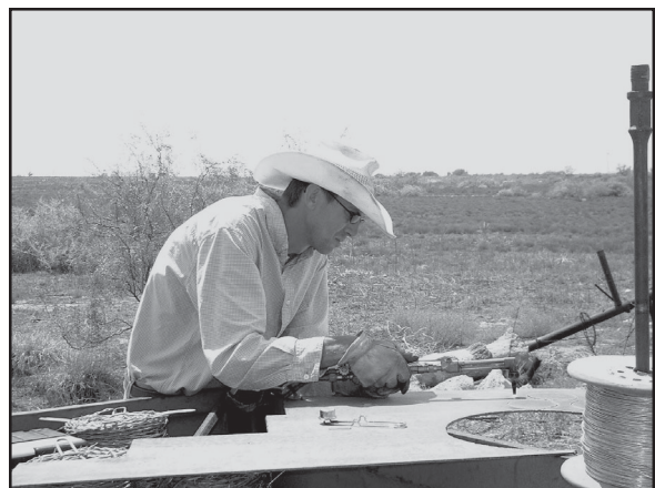
Historic Maintenance Supervisor Scott Trevey works on rebuilding the Landmark’s northern perimeter fence.
